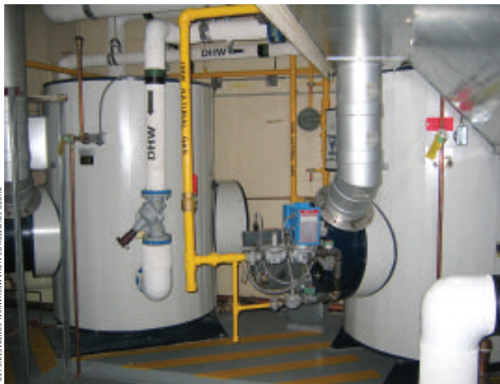
Two new energy-efficient hot water tanks supplying domestic hot water to the existing 820,000-square-foot Domestic Terminal Building at YVR.
