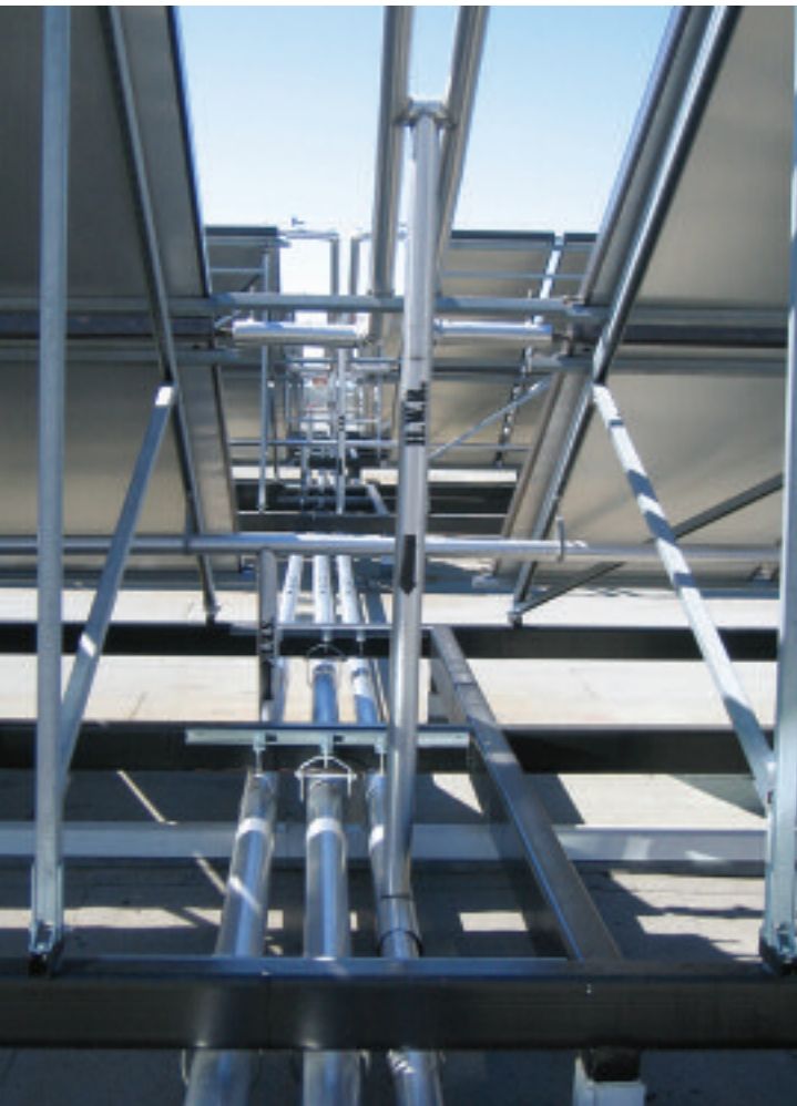
PHOTO COURTESY OF ALPHA MECHANICAL CONTRACTING LTD.
