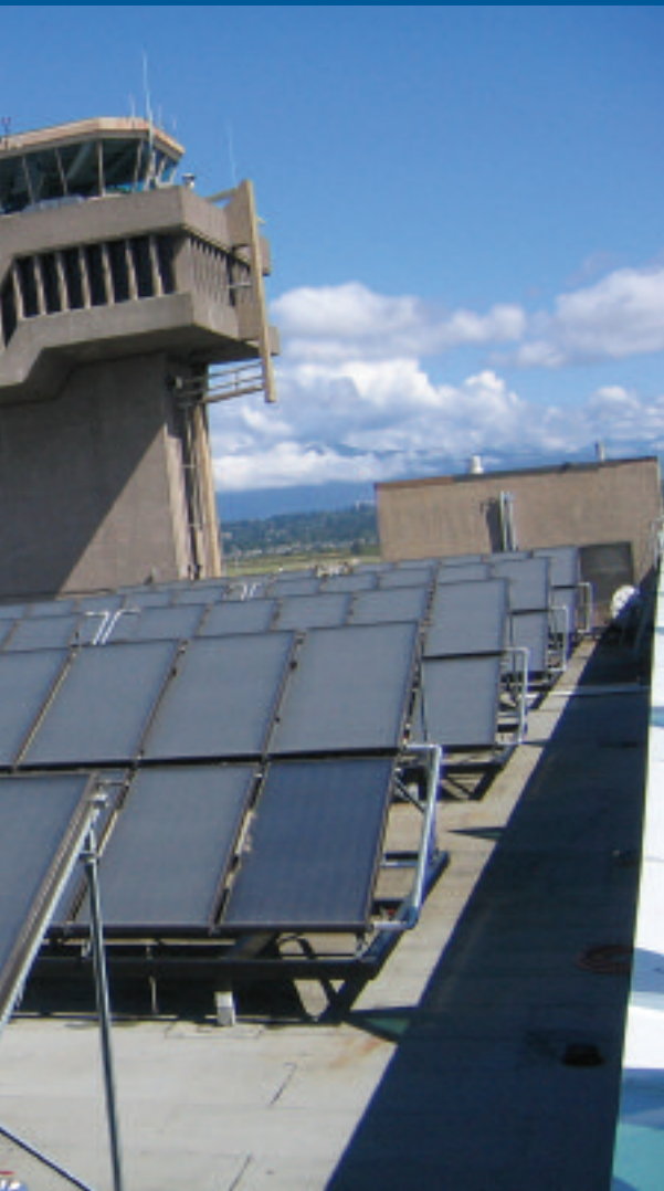
PHOTO COURTESY OF ALPHA MECHANICAL CONTRACTING LTD.
