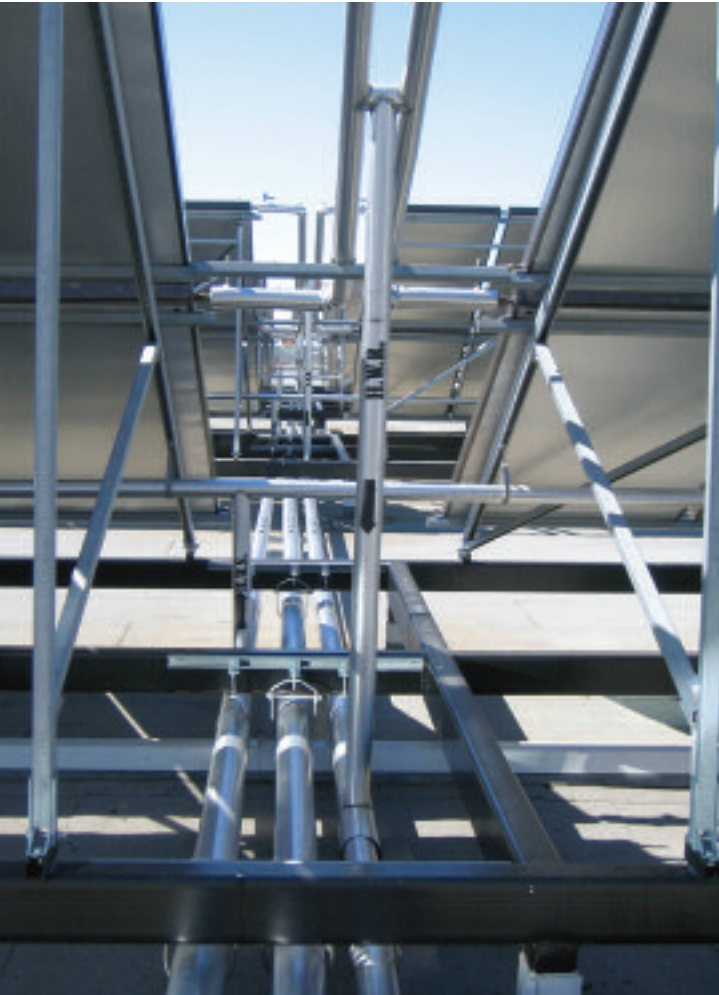
PHOTO COURTESY OF ALPHA MECHANICAL CONTRACTING LTD.
