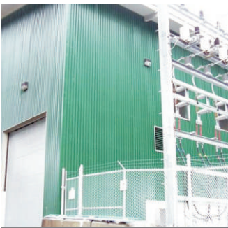
Miller Creek Hydro Electric
