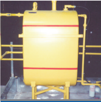
Port Moody Pump Station
