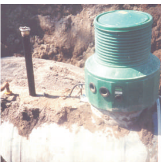
Port Moody Pump Station
