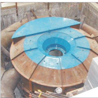
Miller Creek Hydro Electric
