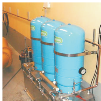
Harbour Pump Station
